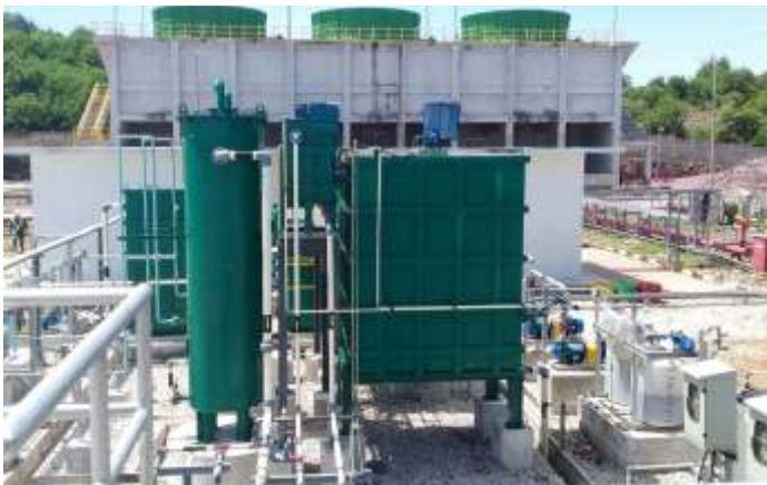
WWTP PLTGU, TG Uncang Batam
