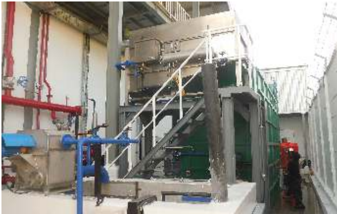
WWTP Diageo, Bali (Beverages Industry, Capacity 5M 3 /Hr)
