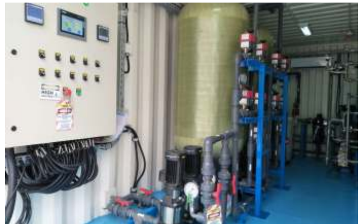
WTP PRETREATMENT ON Container PLTMG Kendari, Jayapura
